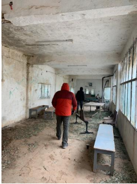
Figure 3: Sample of Jerash Nursery buildings require refurbishment
